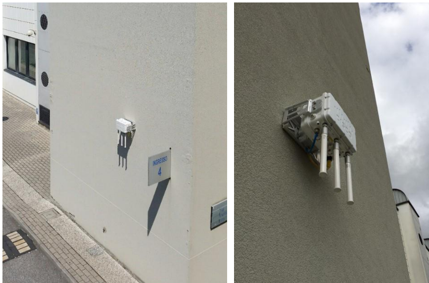
Wall mounted access point
